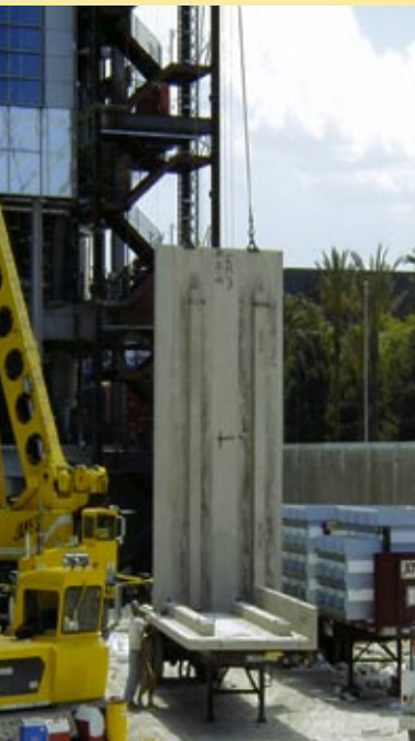
Fig. 8 – The 6 in. thick x 22 ft. tall panels were reinforced with ribs spaced 6 ft. apart.
